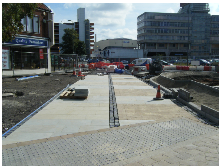
Looking east towards Anglia Square showing the new paved area outside the Wallace King store
