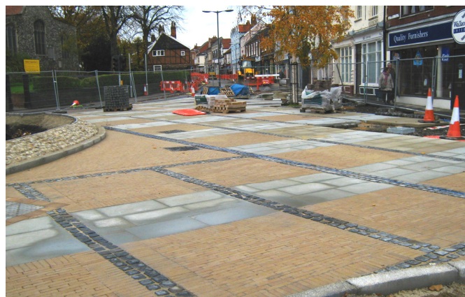
The landscaped area outside the Wallace King store, which is nearing completion
